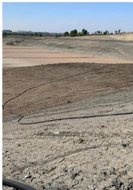
Example of Gas Scavenger Lines Deployed in Phase 12
